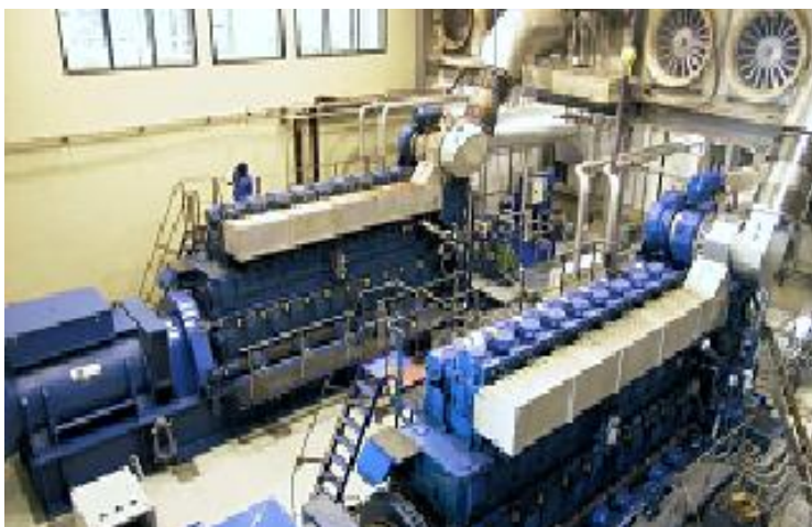
Figure 21: UNELCO Generators in Port Vila running on coconut oil fuel blend (Source: UNELCO).
