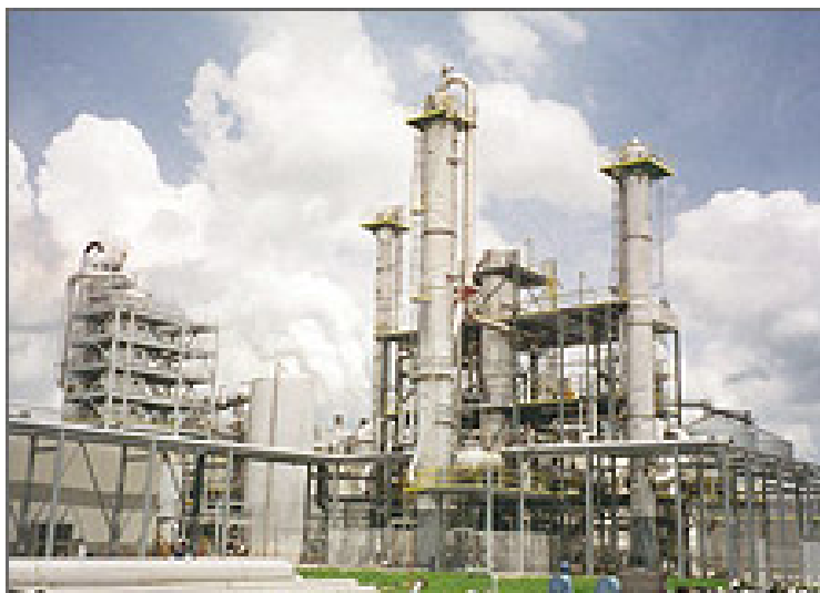
Figure 13: Ethanol Plant with distillation columns (Source: US Department of Energy, Chris Standlee).
