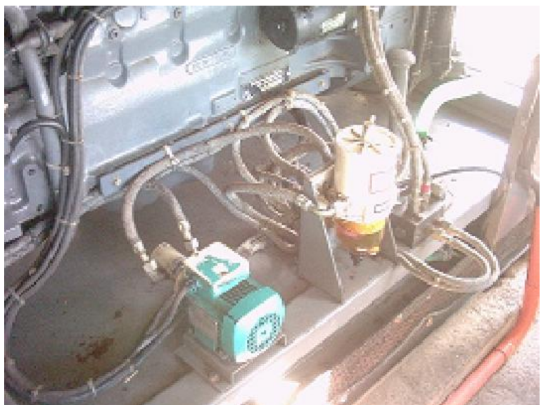
Figure 4: Dual fuel system in Fiji, Welagi community generator (Source: SOPAC).
