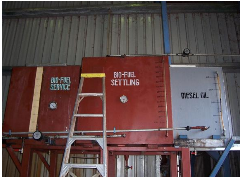
Figure 23: KCMC copra mill in Kiribati uses coconut oil blended with kerosene in their production boilers (Source: SOPAC).
